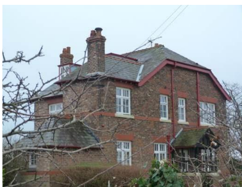
Ash Farm House, with the characteristic National Trust red rainwater goods and bargeboards
